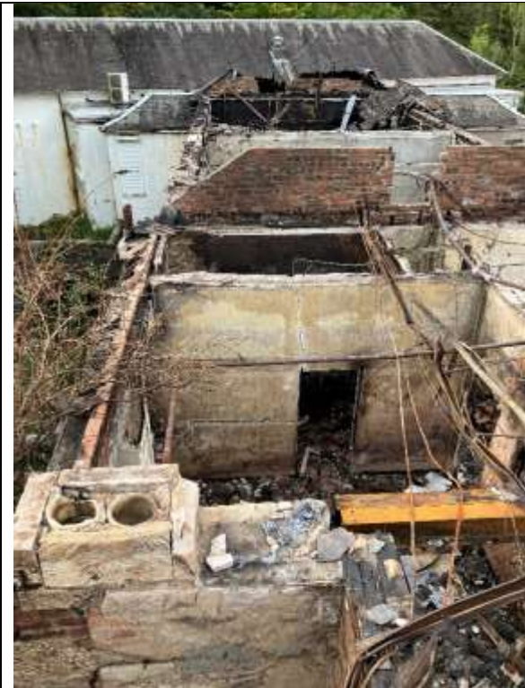
Movement and Cracking of Cross Wall
