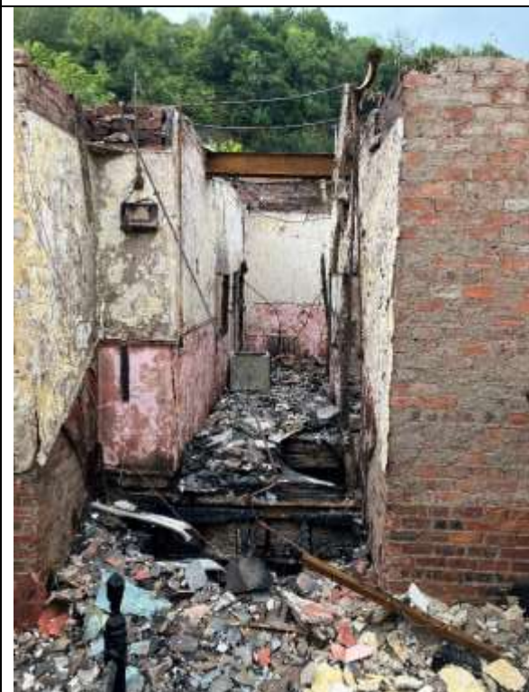
Corridor Looking South Showing Movement
