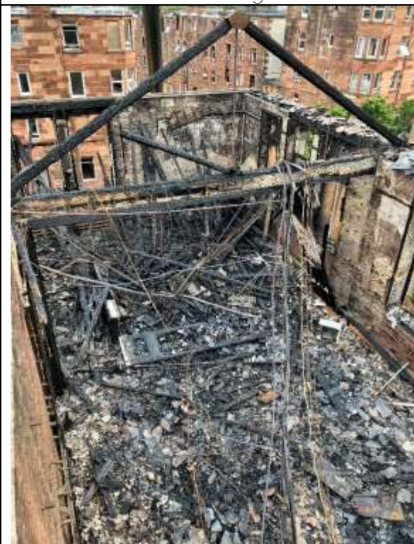
Roof Debris in North Wing
