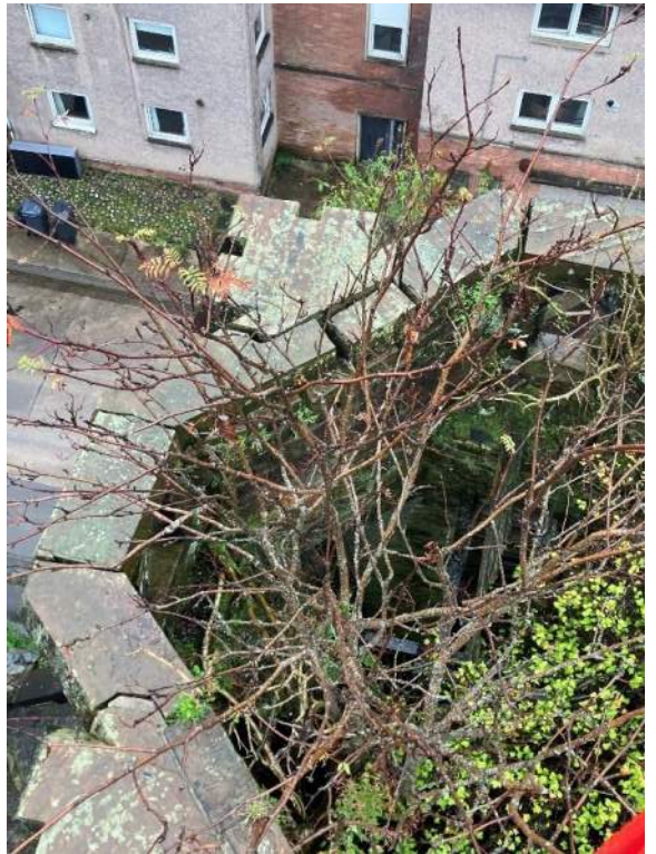
Movement of Stone Parapet
