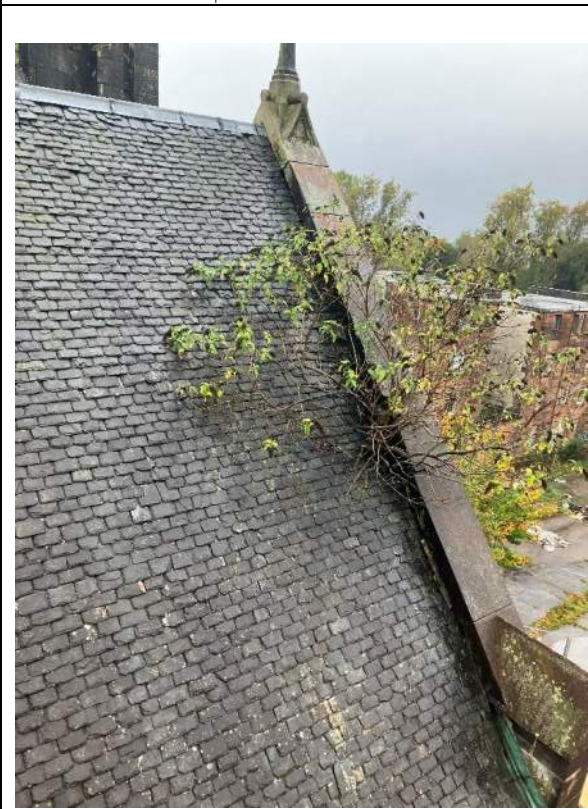
Tree Growth and Missing Flashing
