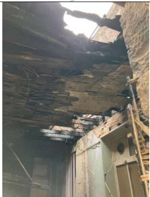
Floor Damage from Below
