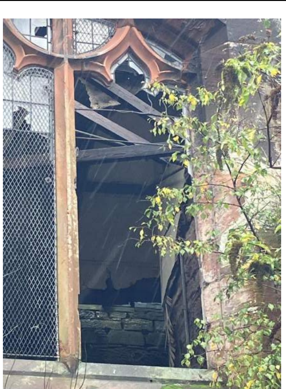
Partial Internal Roof Collapse
