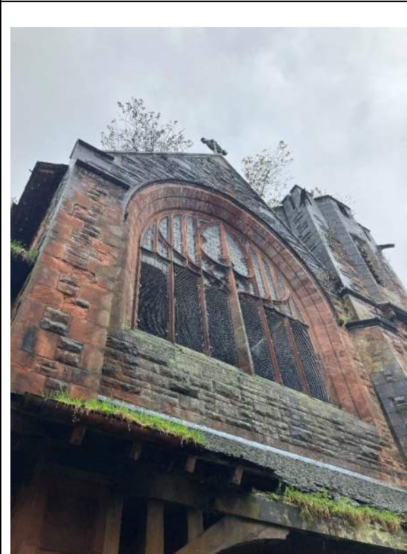
North Elevation with Canopy Damage
